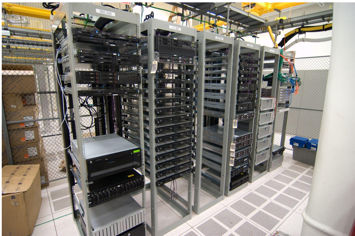
Rack containing servers
