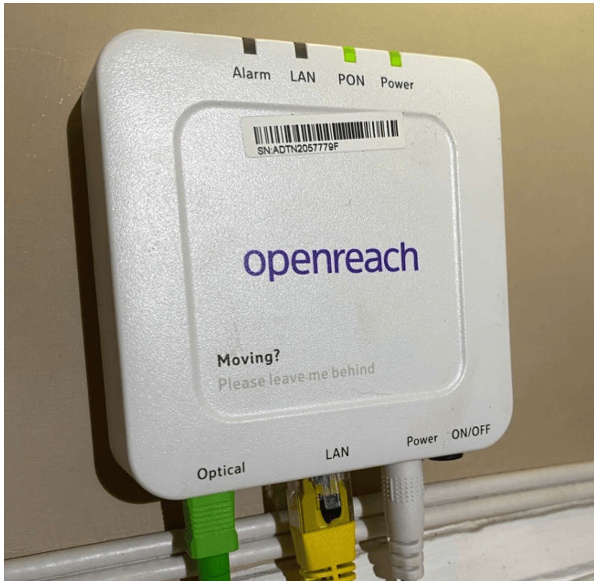
An ONT. Notice that a digital signal enters through the LAN cable—the local network—and an optical signal exits through the optical cable.
