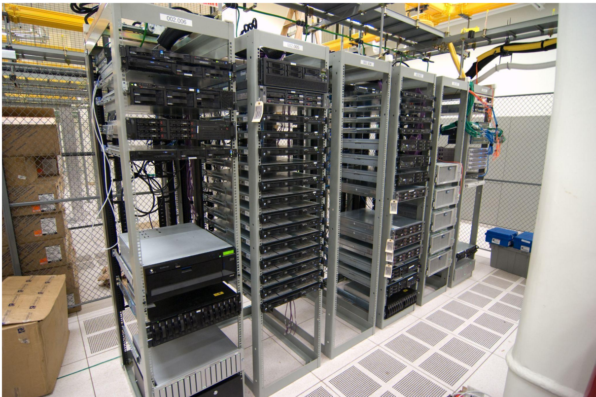
Rack containing servers
